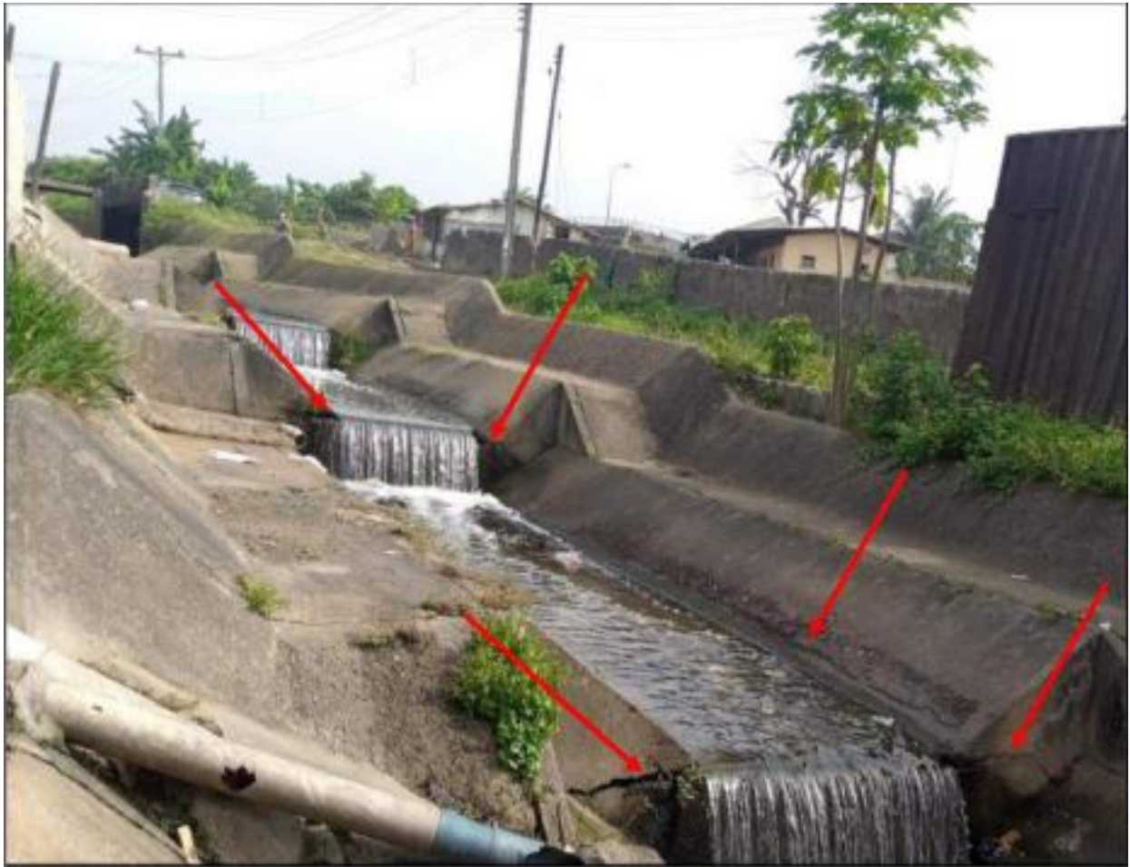
Fig. 2.2S Examples of cracks within the concrete WDO in Okochiri.
